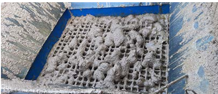
Drilling sludge preparation unit
